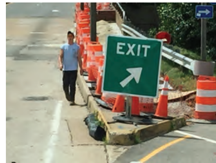
Improper accommodation of pedestrians in a work zone
